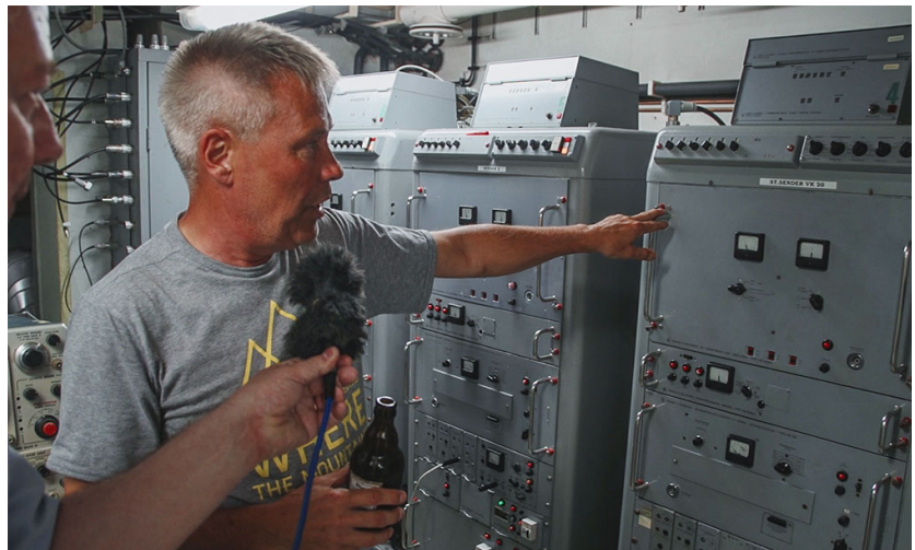
Chief engineer Burkhard with the current 6085 kHz TX. (Left and right: 6005 and 3985 kHz)
