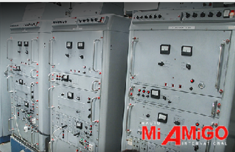
The transmitters in Kall, Germany
